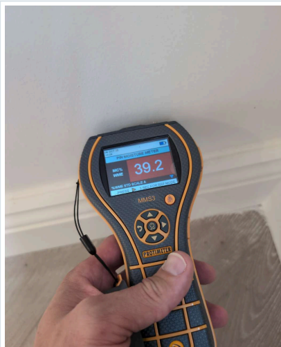
DEFECT External wall left of front window
