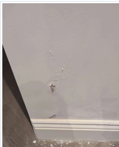
DEFECT Internal partition wall to living room
