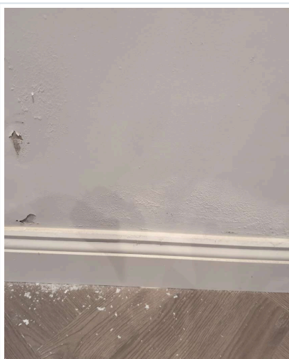
DEFECT Internal partition wall to living room
