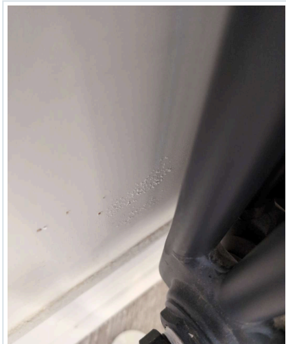
DEFECT Salting signs behind front wall radiator
