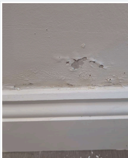
DEFECT Side external wall
