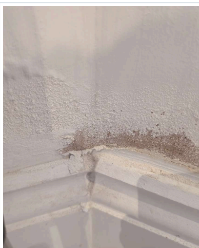
DEFECT Side external wall
