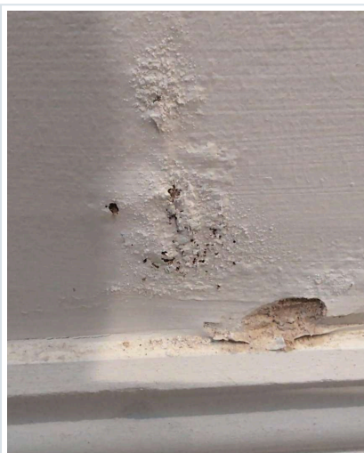
DEFECT Side external wall
