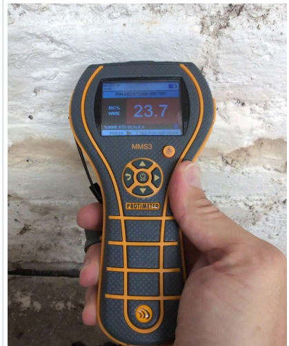
METER IN POSITION
