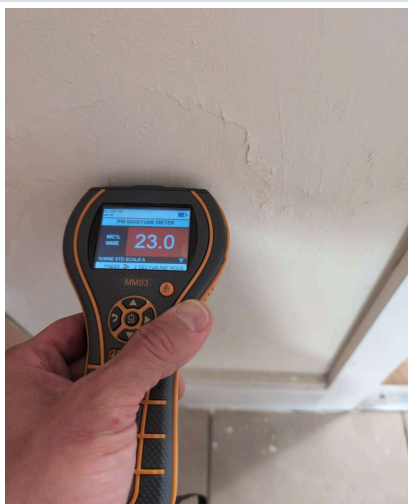
METER SHOWING THE READING
