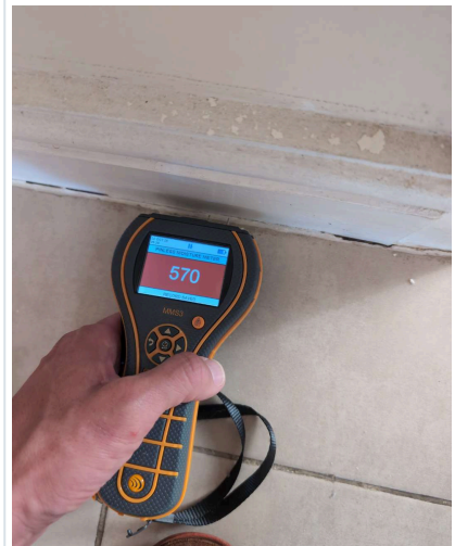
DEFECT Pinless reading on the floor at the foot of the wall
