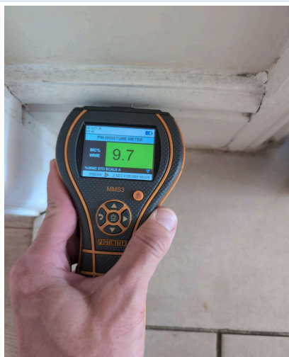
METER SHOWING THE READING
