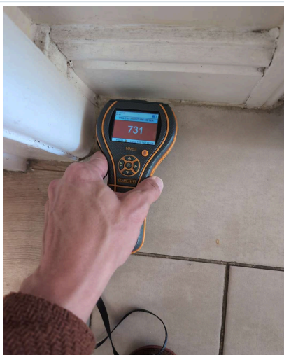
DEFECT Pinless reading at the foot of the wall right of the door
