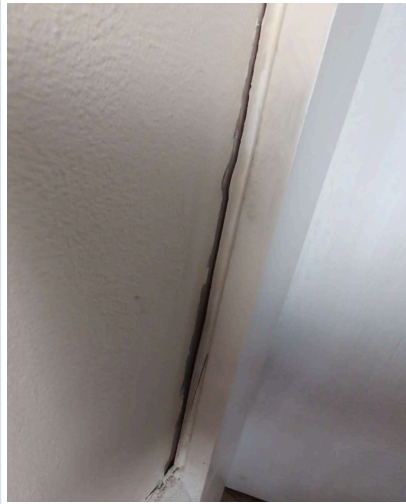
DEFECT Damage directly above the radiator valve
