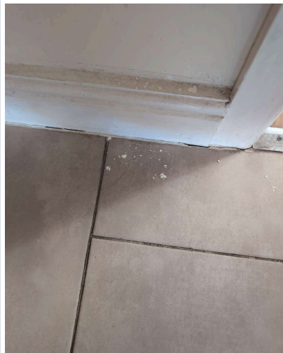
DEFECT Plaster debris on the floor tiles at the foot of the wall
