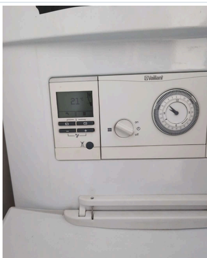
DEFECT The boiler, which the owner reports has to be topped up regularly
