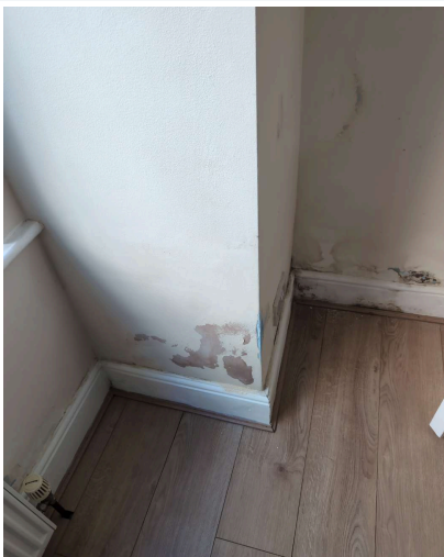
DEFECT The old chimney breast
