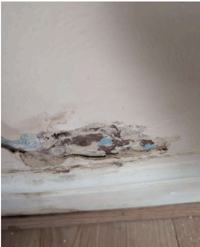
DEFECT Blown plaster and staining above the skirting
