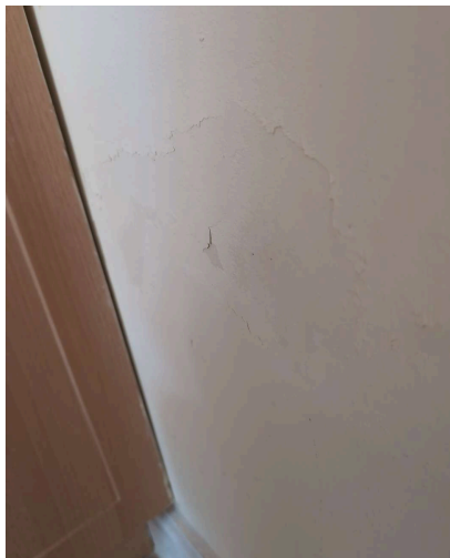
DEFECT Kitchen side: soft, crumbling plaster left of the living room door
