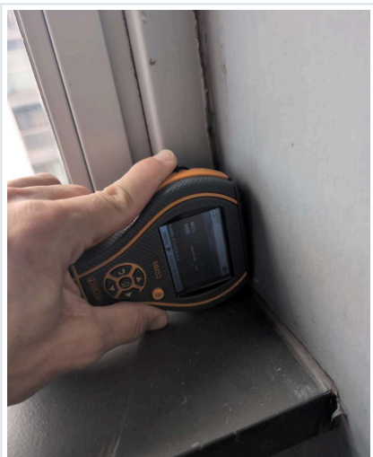
METER SHOWING THE READING
