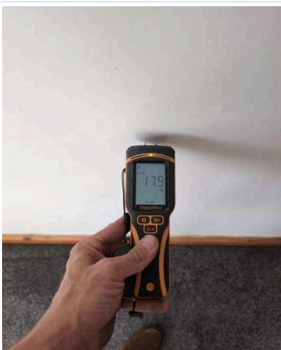
DEFECT West external wall
