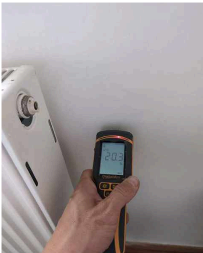
DEFECT South external wall
