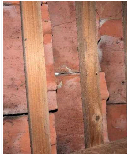
DEFECT Gap in tiles course
