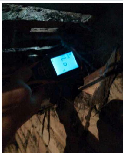
METER SHOWING THE READING
