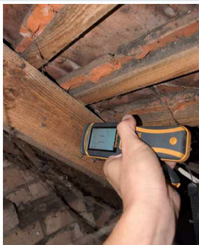
METER SHOWING THE READING
