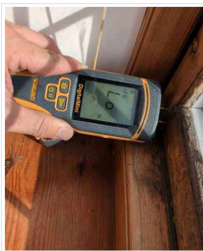
DEFECT Window frame south elevation
