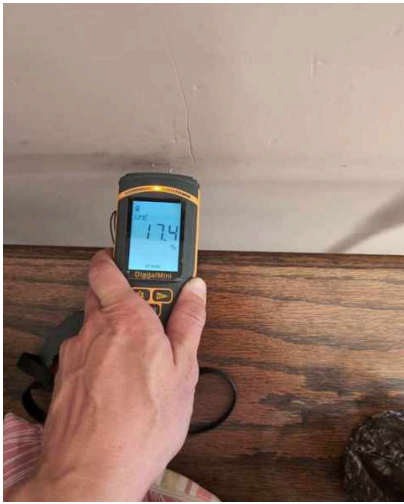
DEFECT South external wall
