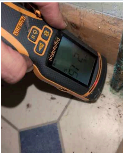
DEFECT Floor reading next to the right hand radiator tail
