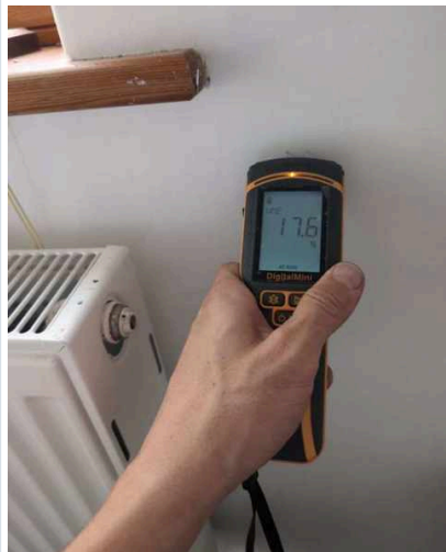
DEFECT South external wall
