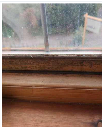
DEFECT Window frame south elevation
