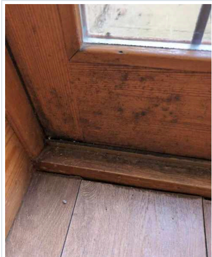
DEFECT Staining to French doors
