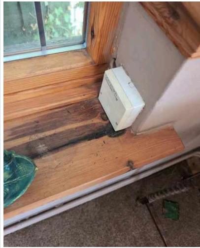
DEFECT East external wall window sill
