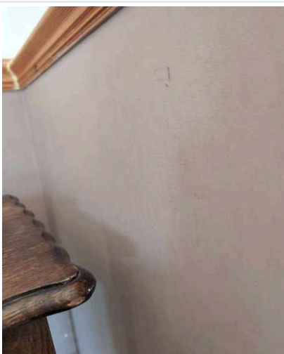
DEFECT East wall, faint marking
