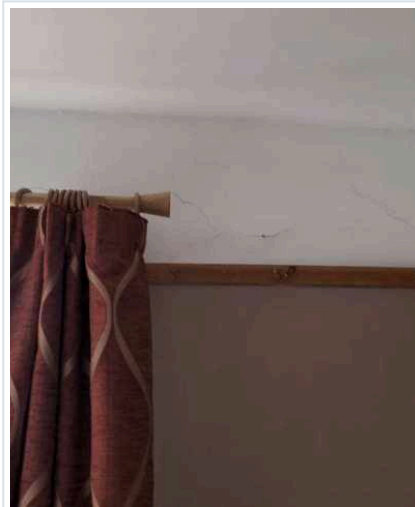
DEFECT External front elevation wall
