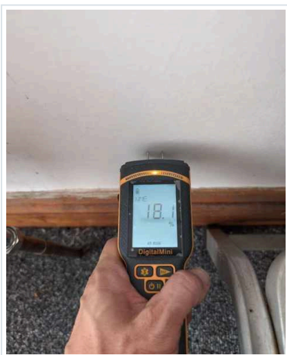
DEFECT South external wall
