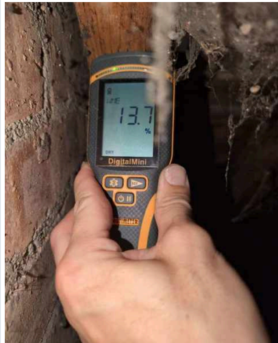
METER SHOWING THE READING
