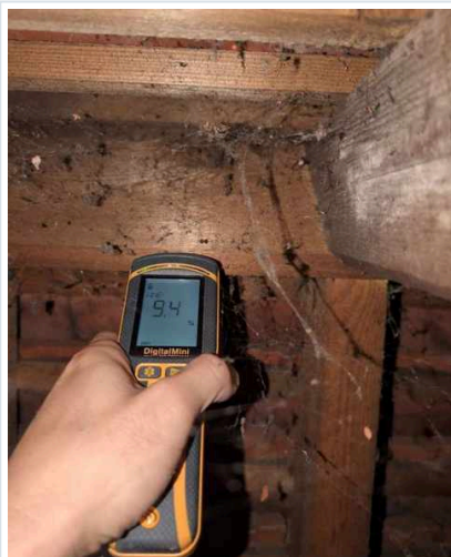
METER SHOWING THE READING
