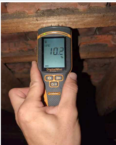
METER SHOWING THE READING
