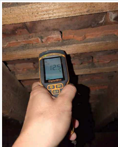
METER SHOWING THE READING
