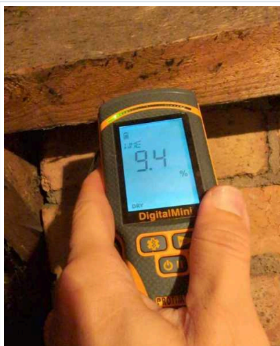
METER SHOWING THE READING
