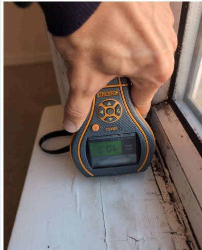
METER SHOWING THE READING
