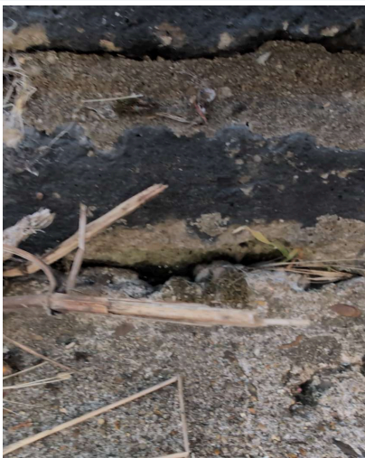
DEFECT Outside, the base of the wall at the cable entry
