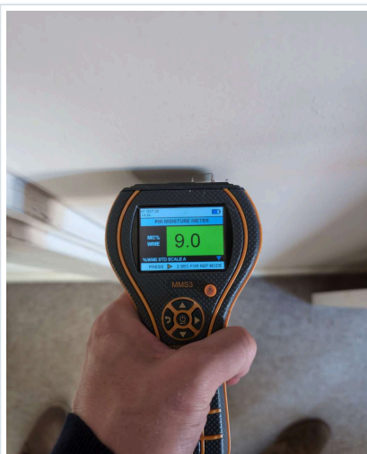
METER IN POSITION
