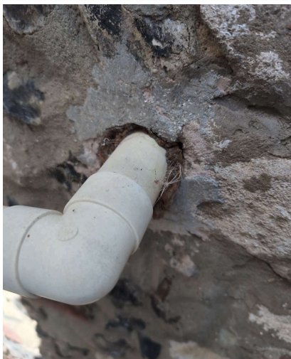
POINTING RENDER Waste pipe through the wall, unsealed
