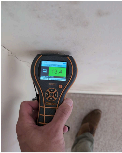
METER SHOWING THE READING
