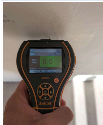
METER SHOWING THE READING
