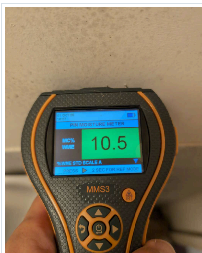
METER IN POSITION
