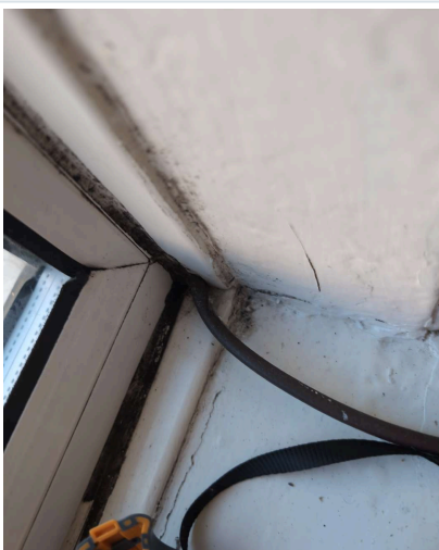
DEFECT Mould to silicone
