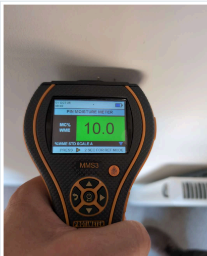
METER SHOWING THE READING
