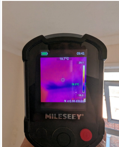
THERMAL Thermal image, cold band at the front wall and ceiling junction
