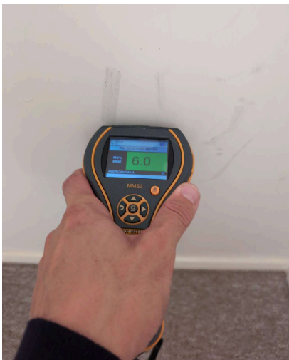
METER SHOWING THE READING
