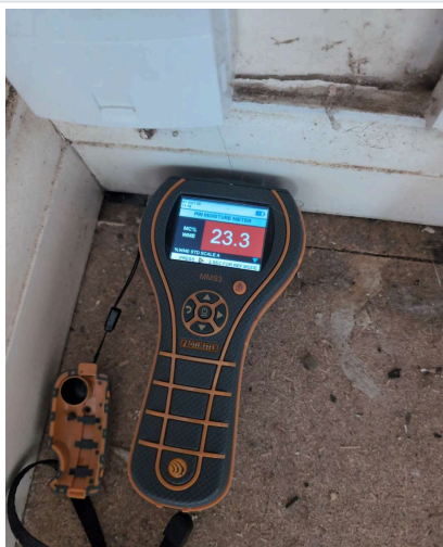
METER SHOWING THE READING
