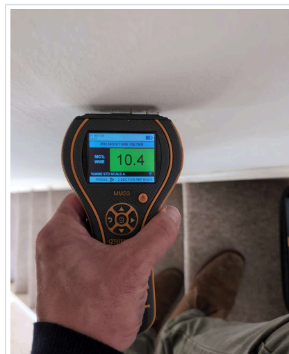
METER SHOWING THE READING
