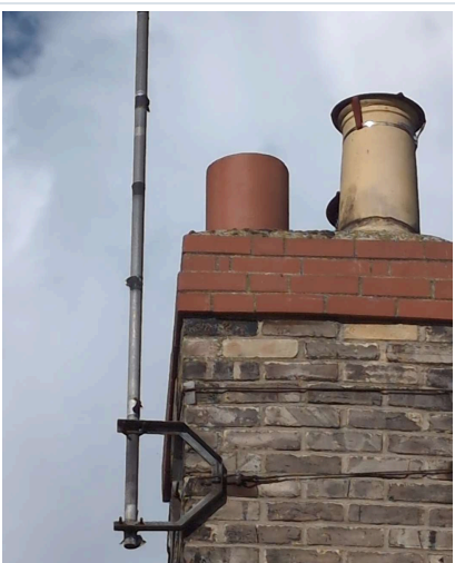
DEFECT Chimney stack, both pots open with no cap
