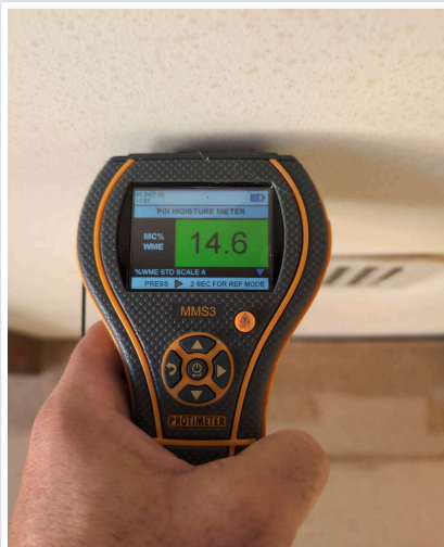
METER SHOWING THE READING
