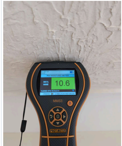
METER SHOWING THE READING
