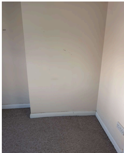
DEFECT Unvented chimney breast
